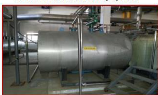
Steam condensate recovery system
