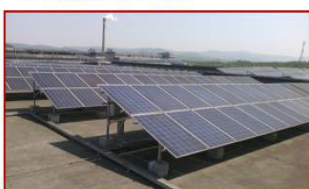
Solar photovoltaic project
