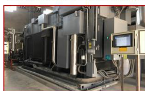
Cooling water waste heat utilization project
