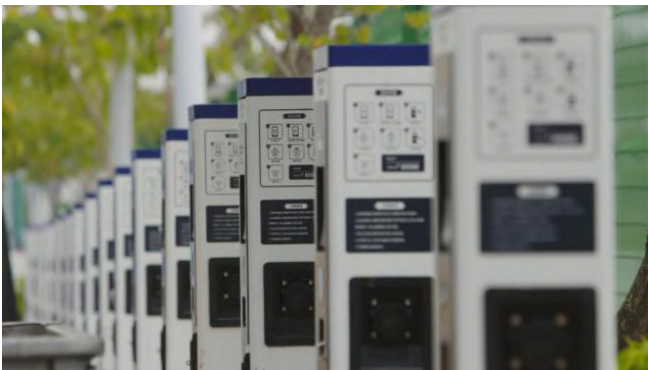
Figure 4 The charging piles
