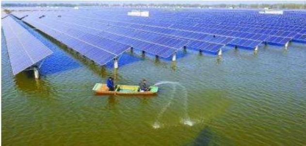
Figure 9 Floating photovoltaic power station
