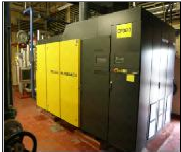
Figure 6: Site Air Compressor with Heat Recovery
