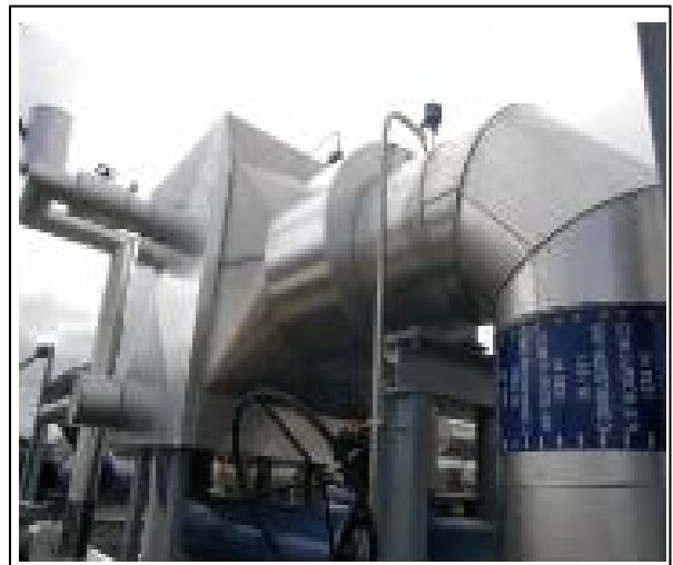
Figure 7: Combustion Air Pre-heater on Incinerator
