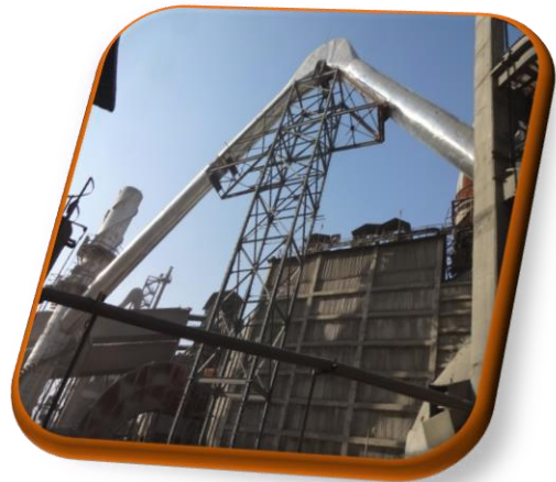
HOT-AIR RECIRCULATION DUCT
